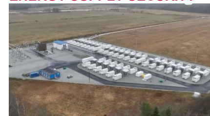
Hertz 1 is the first of two energy storage parks of Baltic Storage Platform. Photo: Evecon
