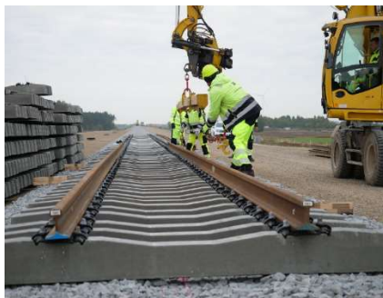
Rail Baltica tracks being laid in the Jona district in Lithuania — one of the fastest-progressing sections of the project. Photo by the Lithuanian Ministry of Transport
